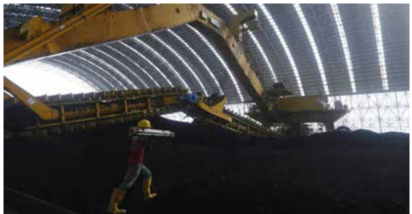
Coal is being stored for the Maitree Super Thermal Power Project near the Sundarbans, the world's largest mangrove forest, in Rampal, Bangladesh
